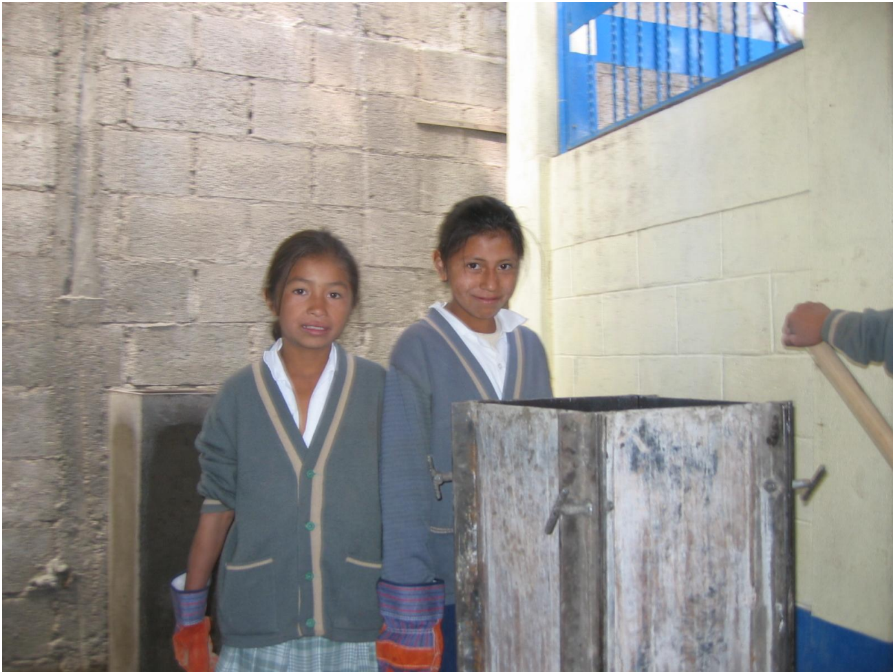
Two Grade 5 Girls Get Ready to Help Fill a Mold with Cement
